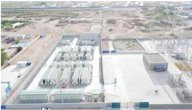
Fig. 10 Grid-forming power storage station in Ejina
